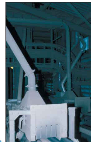
Dust extraction system in a mineral processing plant
